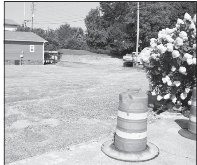
The next step for the newly leveled parking lot at Blairsville City Hall is paving, which should begin soon. Photo by Shawn Jarrard
